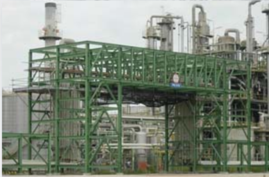
ATC PIPELINES RAYONG
