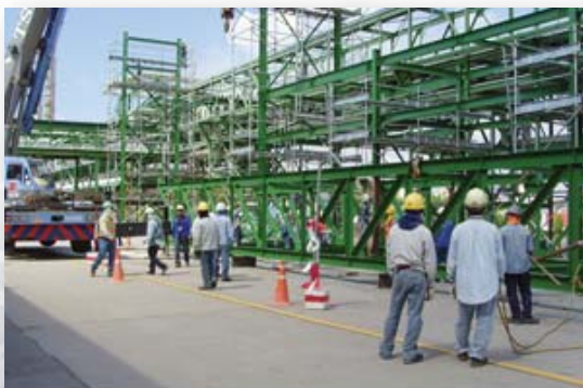
PTTCHEM PIPE RACK RAYONG
